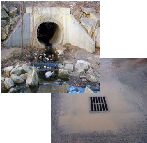
Above - the black substance indicates a potential illicit discharge.
